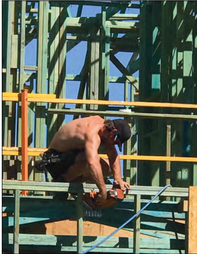
Construction worker with no hard hat, no gloves, no safety boots, or fall prevention. Photo: M Santos
